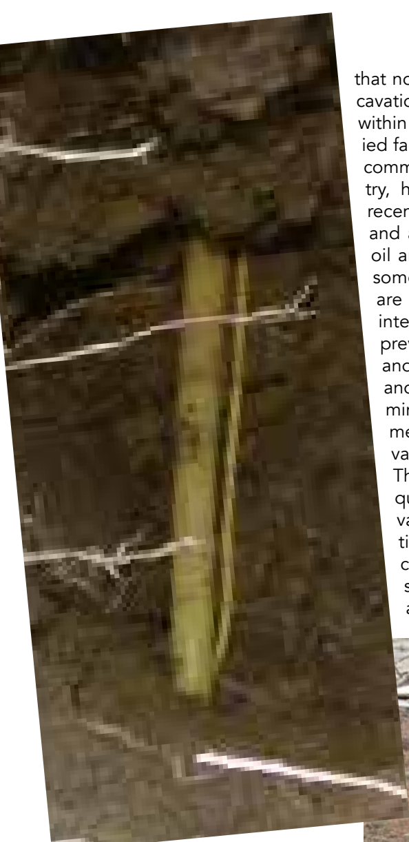
An exposed plastic gas service and tracer wire.
