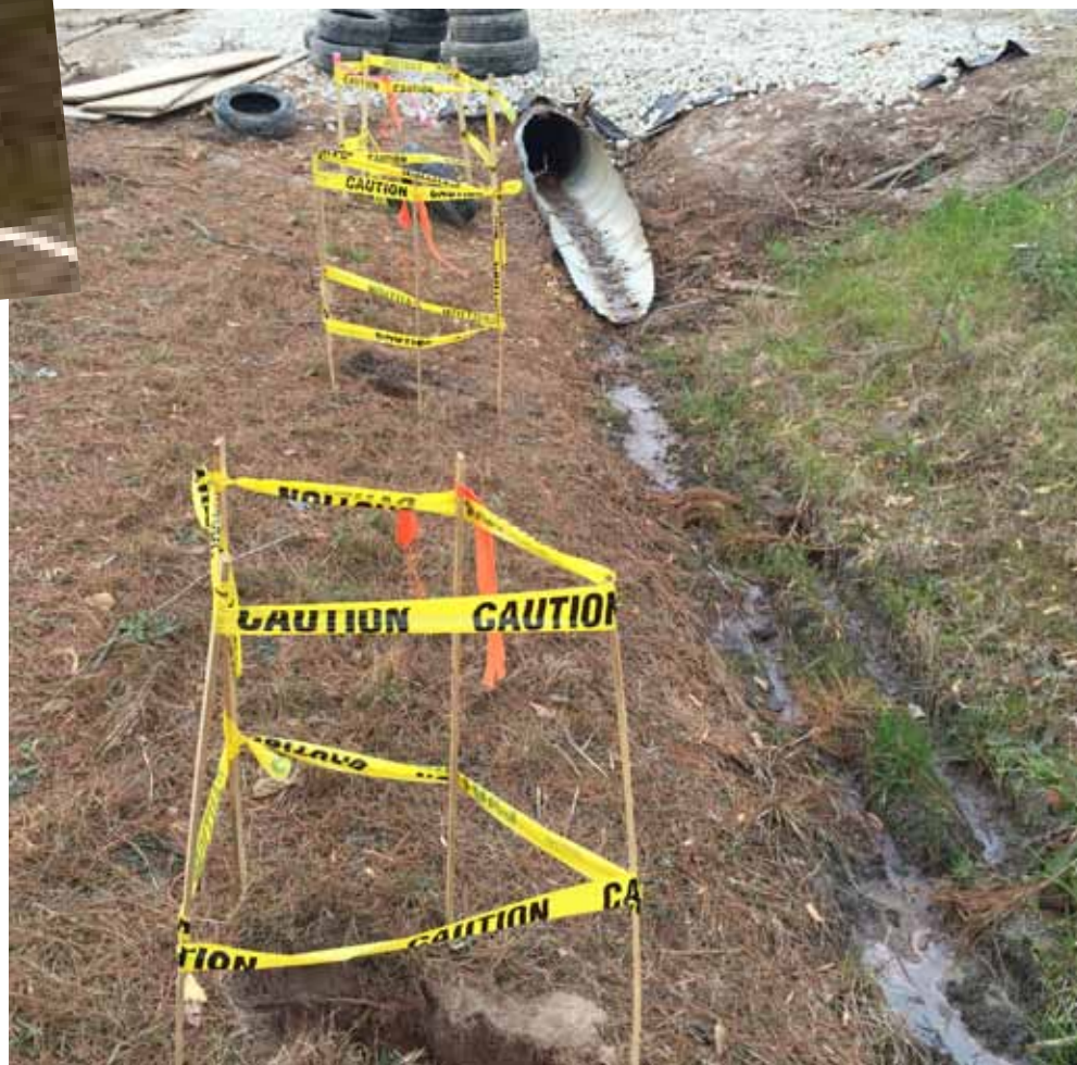
Three pot holes have been made along the path of this buried utility, meaning it could be intersecting another line somewhere down the path.
