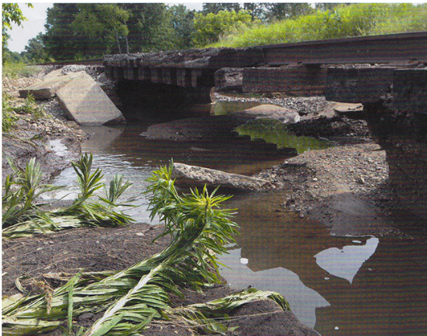
Erosion and flooding can cause damage missed by aerial patrols 1,700 feet or more in the air. Comprehensive ground right-of-way patrols by trained technicians can spot such damage before a rupture occurs. Source: Atlas Field Services LLC
